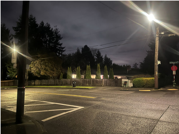
Existing LED Streetlighting SW Trenton Street
