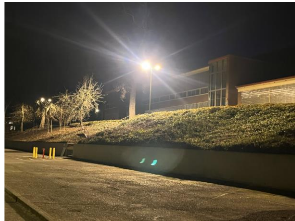
Existing LED pole mounted parking lot lighting
