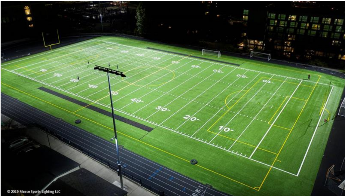
Roosevelt HS LED Lighting System
