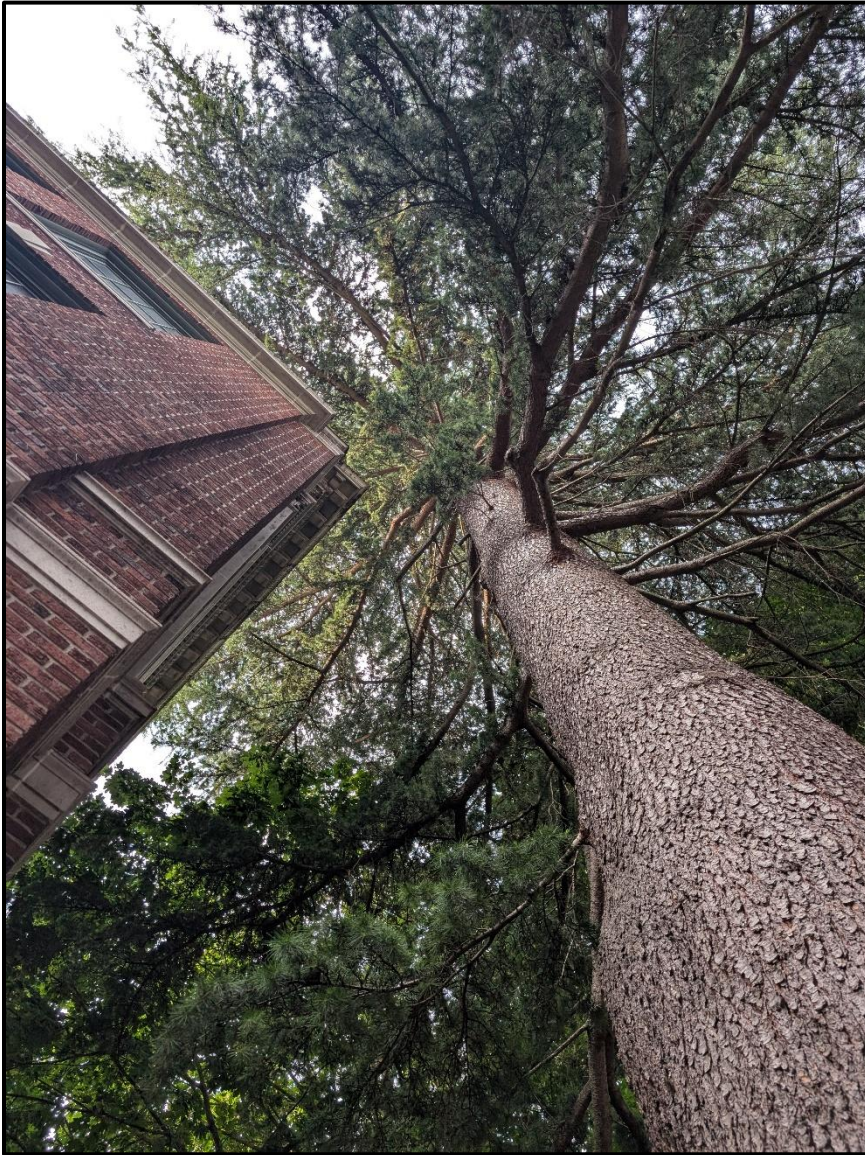
Photo 3. Looking up at tree 350. If the building needs masonry repairs, clearance pruning may be needed.
