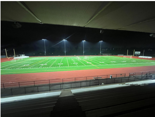
Existing Football Stadium Lighting
