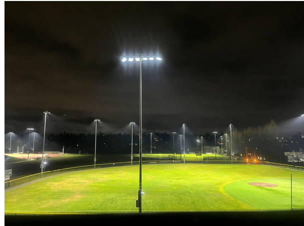
Existing Baseball and Softball Field Lighting
