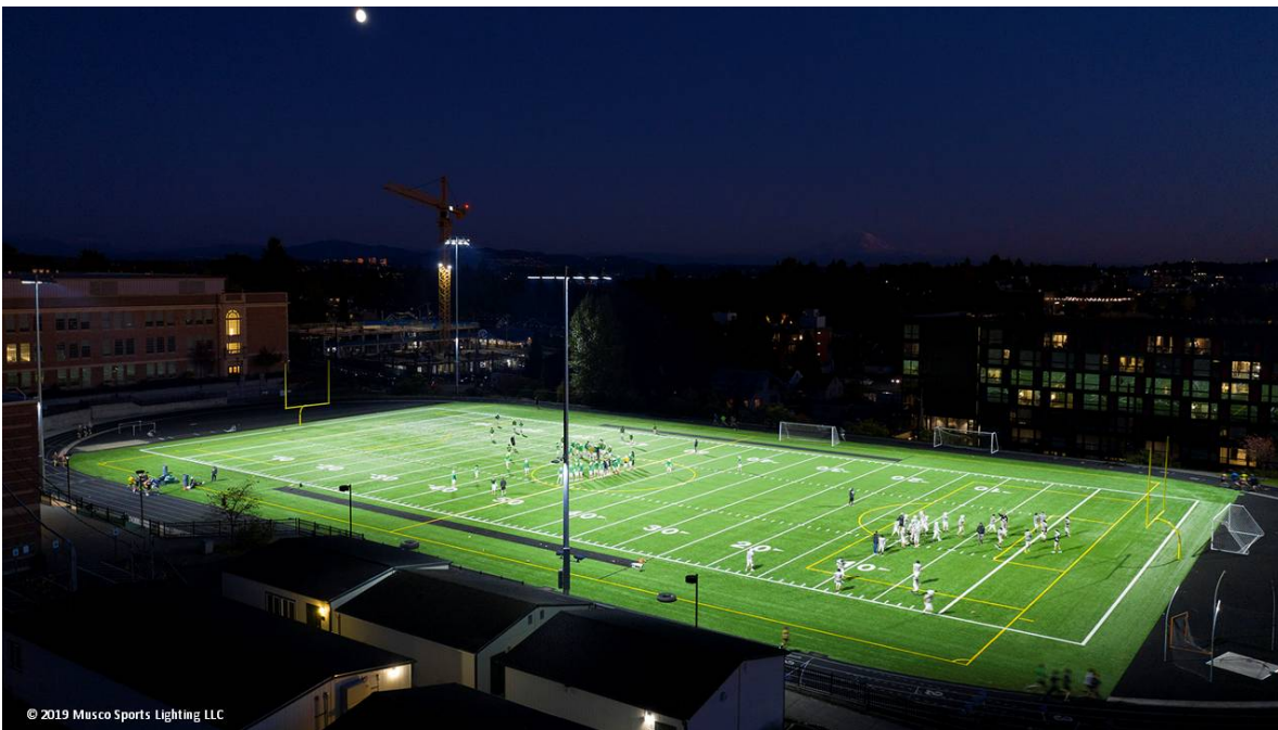
Roosevelt HS LED Lighting System
