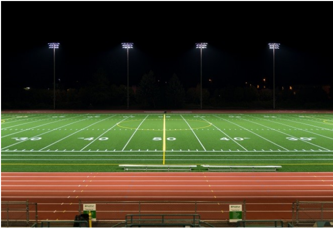
Direct glare reduction with use of advance shielded LED floodlights
