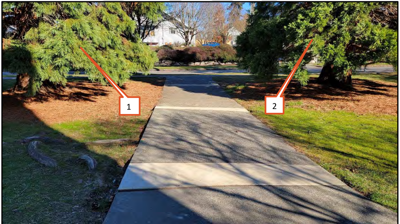
Photo 2. View looking to the north at the base of trees 1 and 2. Structural roots have been cut at the walkway where conflicts have occurred. Future walkway repair should consider alternative methods prior to root removal.
