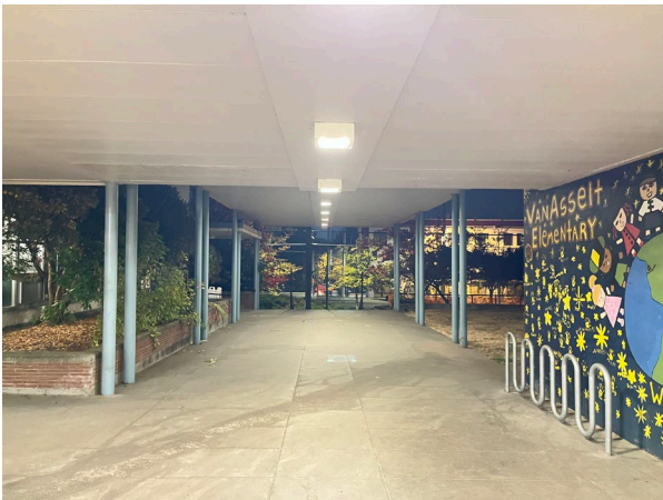
Existing LED school east entry lighting
