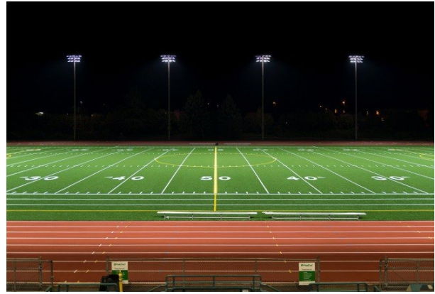
Direct glare reduction with use of similar LED floodlights
