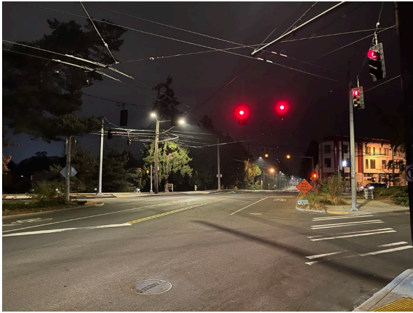
Existing Intersection Lighting Beacon Avenue South
