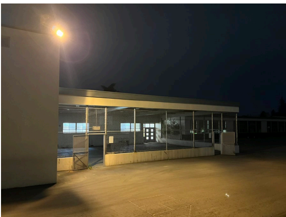
Existing HID building mounted floodlight lighting
