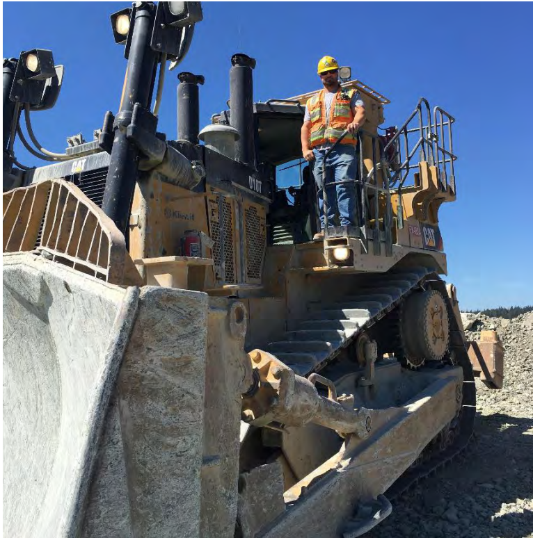
Photo: Steven Neese (2yr Apprentice) taking a moment from his busy day running a D10 dozer for Kiewit Construction at a rock quarry in Skagit County.
