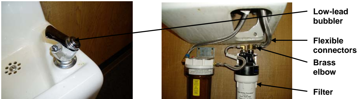
Type C. Typical new bubbler, new flexible connectors and shut-off valve, POU filter system, and brass elbow connectors.
