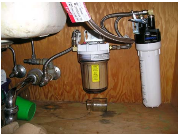
Figure 1. Typical filter installation under a classroom sink, which includes a pre-filter and charcoal cartridge filter connected from the service line to fountain bubbler head (not shown).
