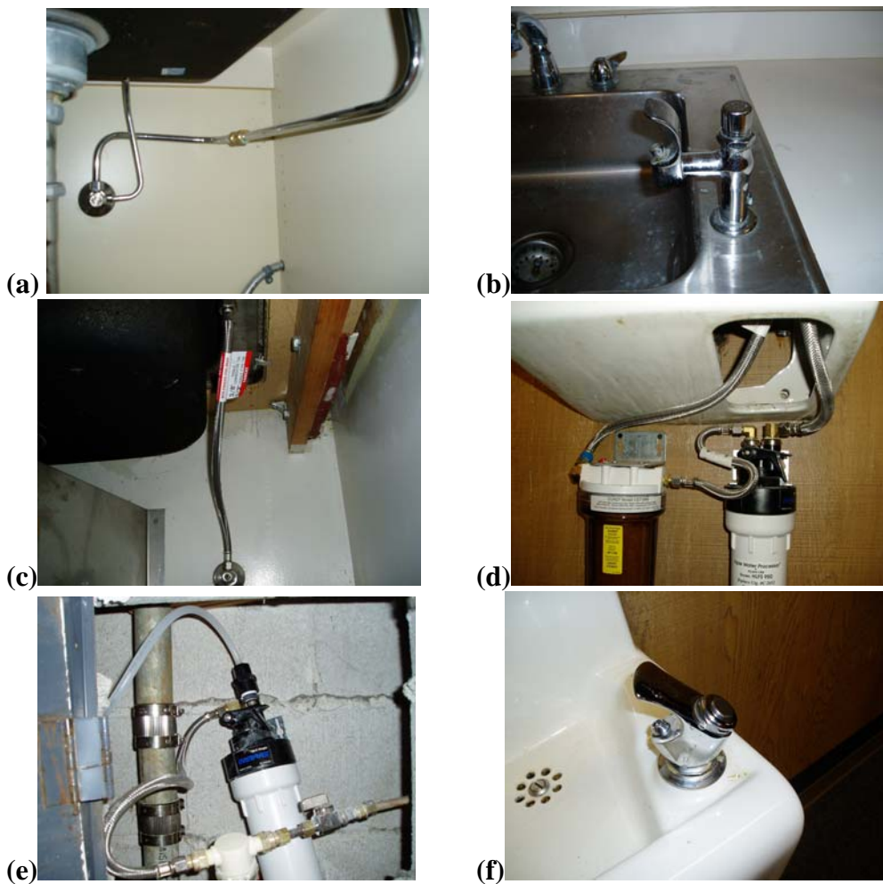
Figure 1. Typical older drinking water fountain installation in Seattle Public Schools showing (a) shut off valve and connective piping and (b) bubbler head and sink. Typical newer drinking water fountain installations showing (c) flexible connective piping with brass ferrule ends, (d) granular-media filter system with flexible connective piping with brass fittings, (e) filter system with plastic fittings and tubing downstream of filter, and (f) low-lead (<0.3% Pb) bubbler head and sink.
